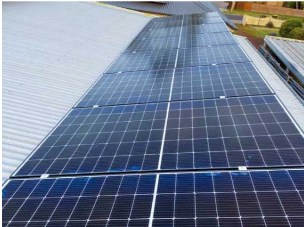
Roof Mounted Solar PVs
