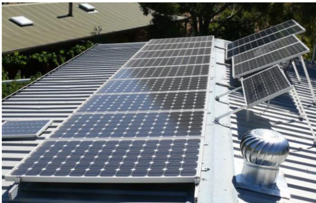
Roof Mounted Solar PVs
