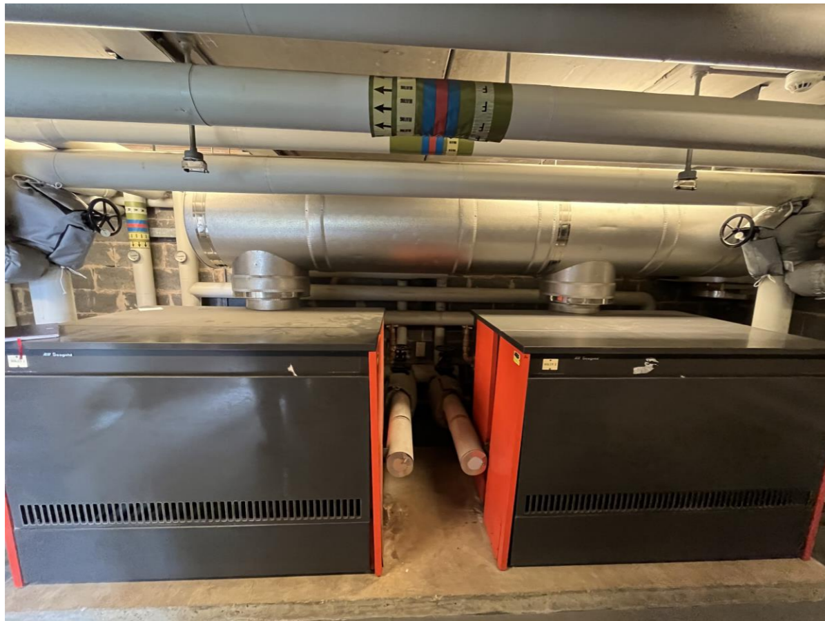
Existing Gas Fired Original Boilers dating from early 90s
