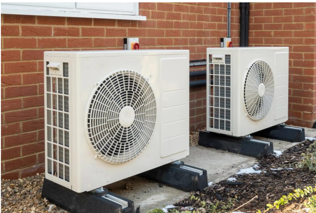
Air Source Heat Pumps
